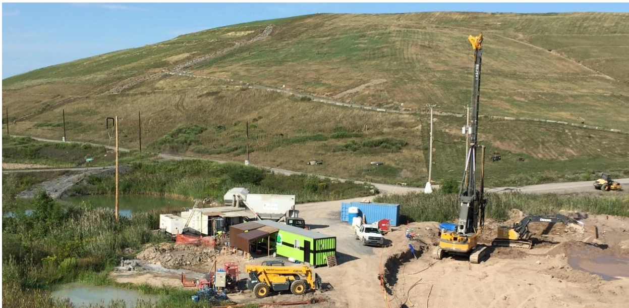
Figure 5. Photograph of Stage 6 site, showing drill rig (right) and batch plant (left)
