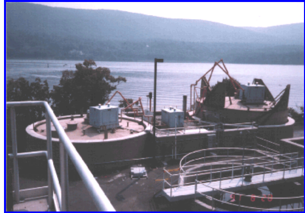
Anaerobic Digesters at Highland Falls STP
